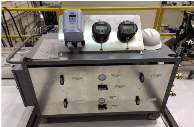
Figure 18: DI Water Fill and Drain Cart.
