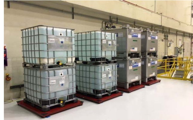
Figure 17: DI and HFE Fluid Storage Totes [9] [14] on Weight Scales [16].
