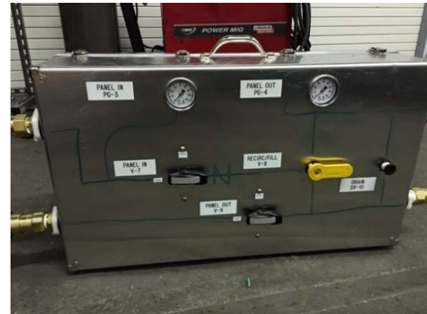
Figure 19: DI Water Portable Panel.
